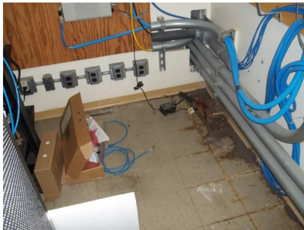
Old Administration Building (101T) – SE Corner Basement Office 6 [9" floor tiles and mastic of 3% Chrysotile]
