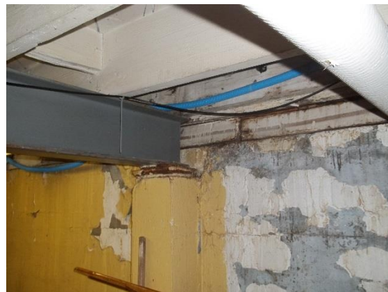
Old Administration Building (101T) – Sample of Old Basement Office Wiring [Area of possible asbestos containing material]
