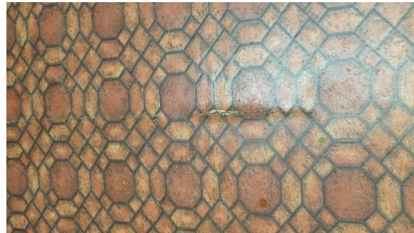
Culture Building (102T) – Floor Covering Crack Detail in Classroom 1 This is original floor covering. [Sheet vinyl flooring with 30% Chrysotile]
