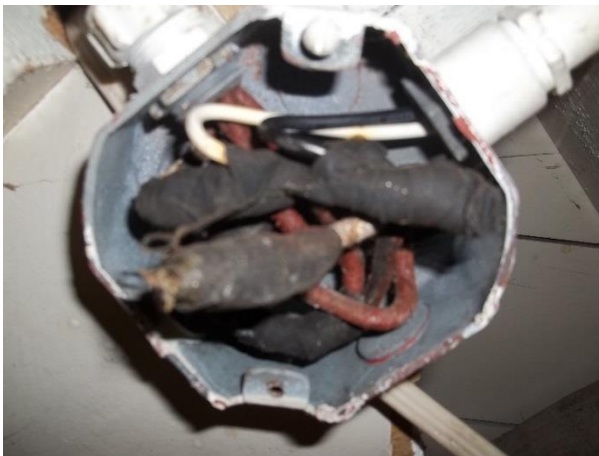
Old Administration Building (101T) – Sample of Old Basement Office Wiring on West End [Area of possible asbestos containing material]
