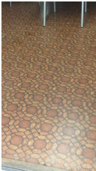
Culture Building (102T) – Floor Covering General Area of Crack in Classroom 1 This is original floor covering. [Sheet vinyl flooring with 30% Chrysotile]
