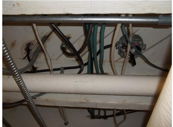
Old Administration Building (101T) – Sample of Old Basement Office Wiring on East End [Area of possible asbestos containing material]
