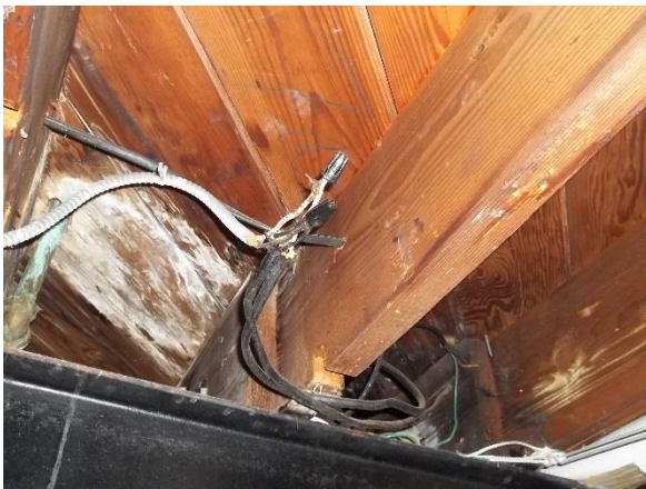
Old Administration Building (101T) – Sample of Old Basement Office Wiring on West End [Area of possible asbestos containing material. WAT 07-29-2016 sample indicated non-asbestos material for a single non-energized wire that is part of picture.]
