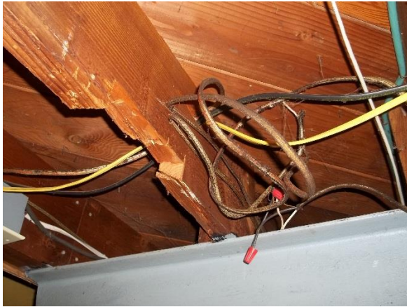
Old Administration Building (101T) – Sample of Old Basement Office Wiring on West End [Area of possible asbestos containing material]
