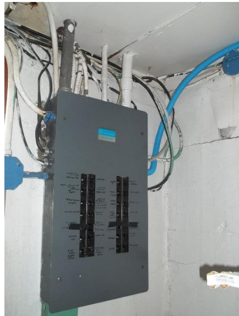
Old Administration Building (101T) – Sample of Old Basement Office Wiring on West End
