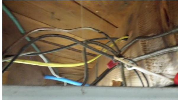
Old Administration Building (101T) – Shop 1 View is looking at assorted ceiling wiring.
