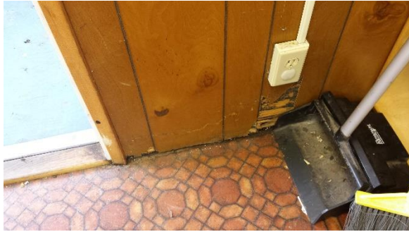
Culture Building (102T) – SE Corner Doorway Detail in Classroom 1 Original floor covering with trim removed and no apparent damage. [Sheet vinyl flooring with 30% Chrysotile]
