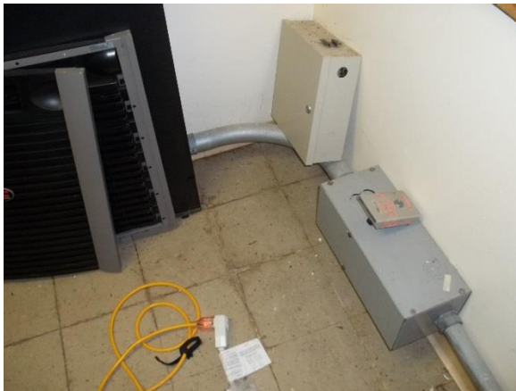
Old Administration Building (101T) – SW Corner Basement Office 6 [9" floor tiles and mastic of 3% Chrysotile]
