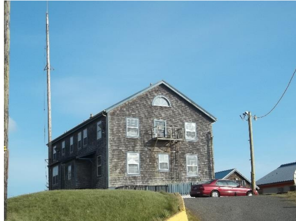
Old Administration Building (101T) - looking East Testing confirmed portions of building contain asbestos.
