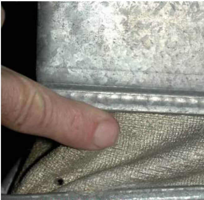
Asbestos fabric in HVAC system
