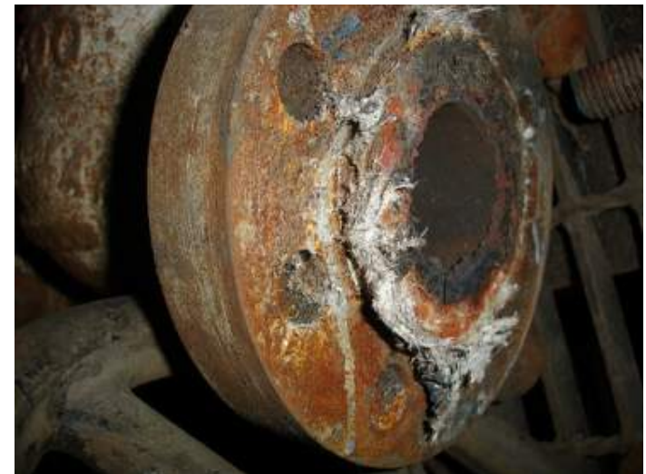
Damaged asbestos gasket
