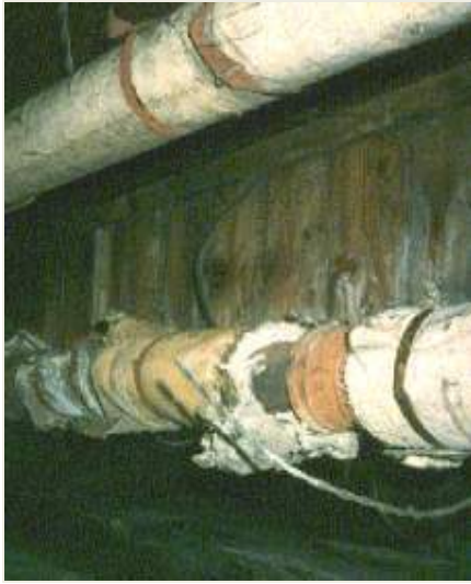
Asbestos insulated pipe
