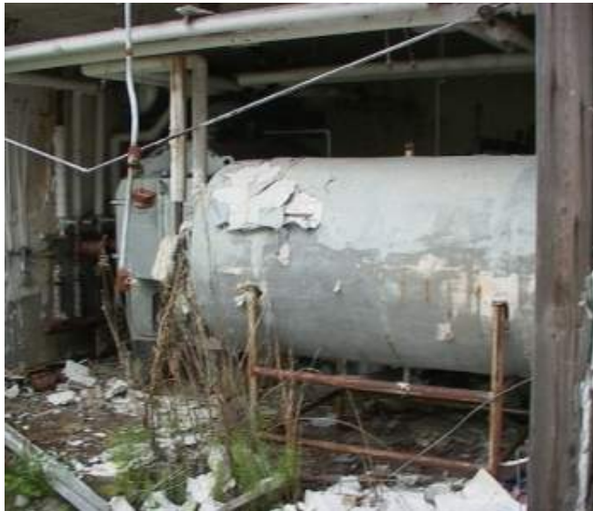
Asbestos insulated boiler
