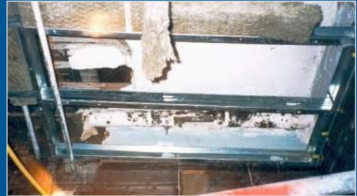
Damaged asbestos pipe insulation
