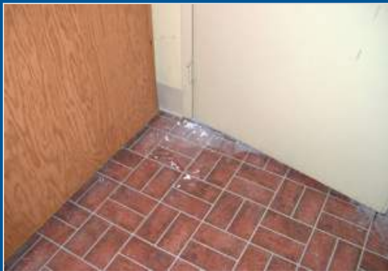
Asbestos debris on floor
