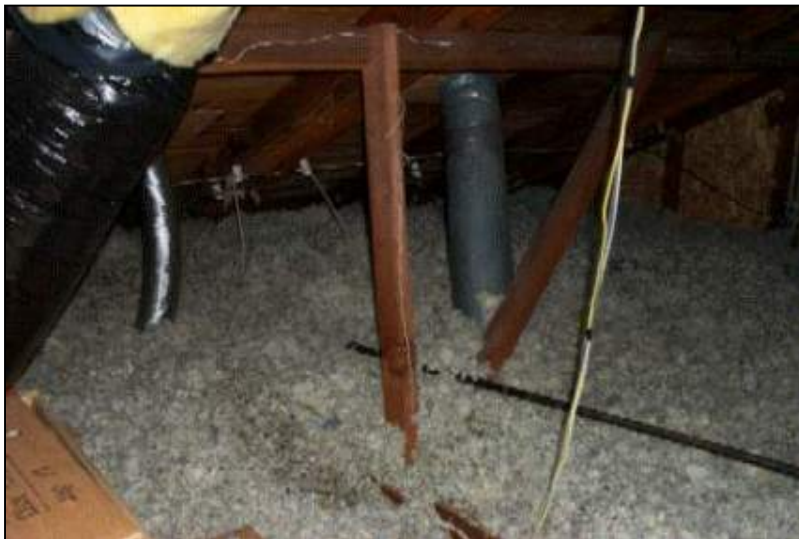
Vermiculite insulation in attics
